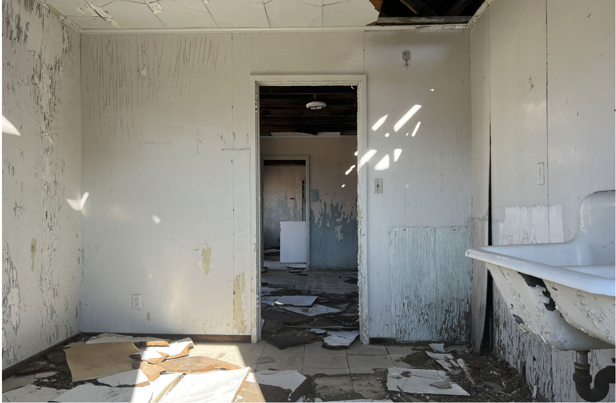
Figure 7. Interior view showing probable lead paint and asbestos contamination.
