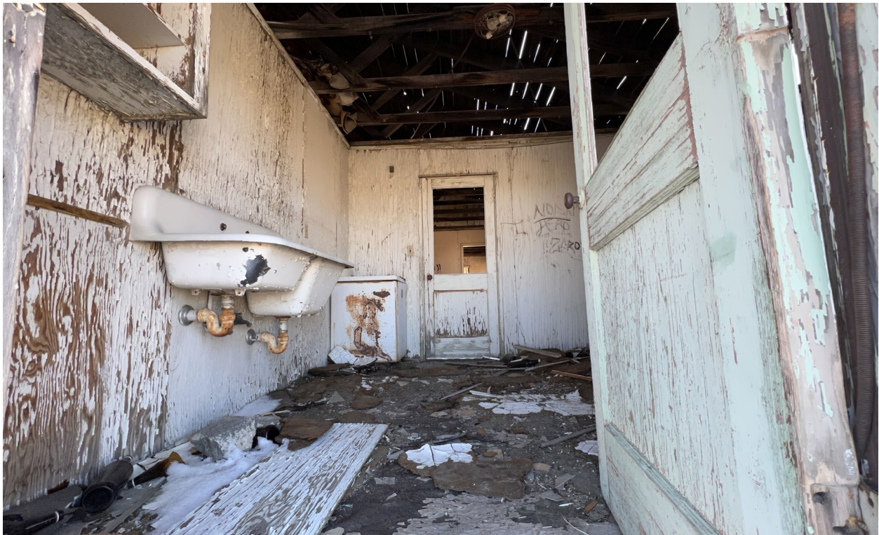
Figure 8. Additional view of the heavily weathered interior and surfaces with flaking paint.
