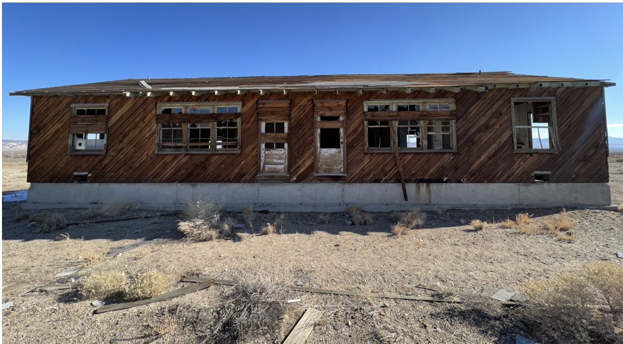
Figure 4. The front of one of the Babbitt house structures as seen looking due east.
